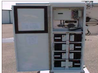
Custom UNI-PAK powers a large and satellite communications link flow meter
